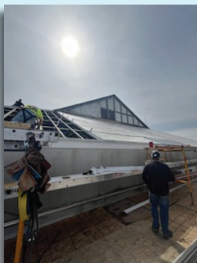
Jen's Glass workers replacing the skylight at ECC City Campus in Buffalo, NY
